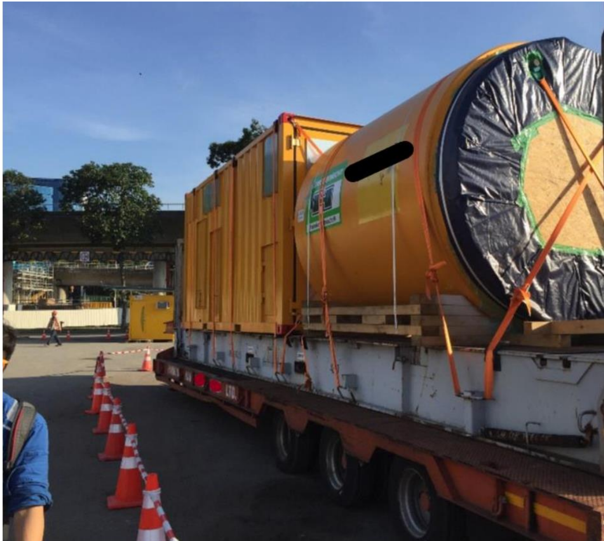
Gantry System. The skip wagons and segments are delivered by a winch system
